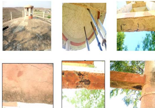
Fig3 Top spherical dome, Bottom spherical slab, Craze cracks, Longitudinal cracks, Spaling of concrete, spalling of concrete
